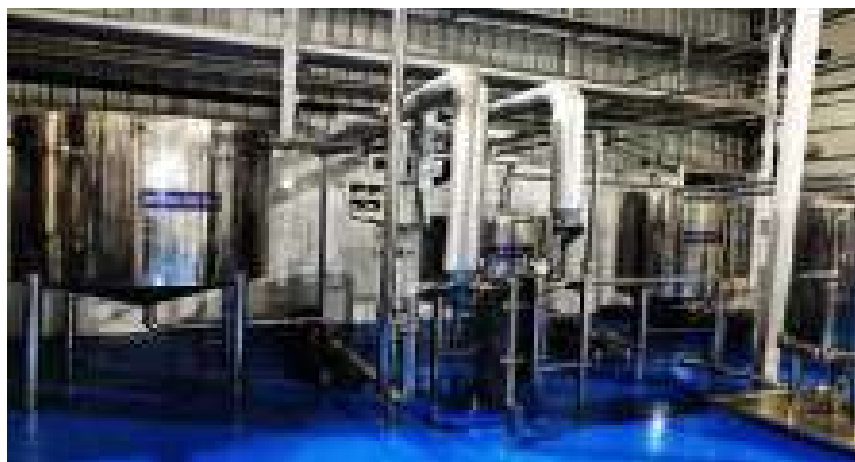
Established a Honey & other beehive Processing Unit under NBHM Scheme at Salt Range Foods Private Limited. Guwahati, Assam
